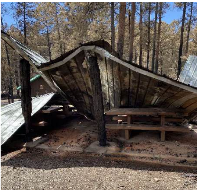
Figure 2: Recreation facility damaged during the fire at Sam Tobias Group Campground
