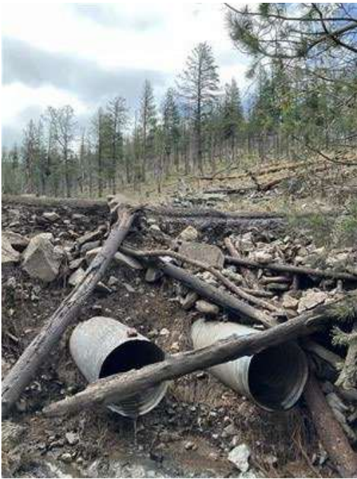
NFSR 127A Roadway Embankment Erosion
